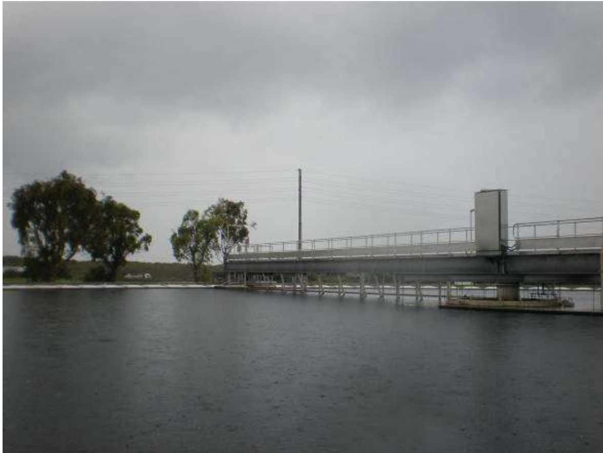
Final Settling Tanks – separates water and sediment.
