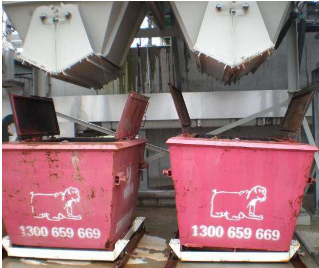
Sludge and waste is emptied during treatment process
